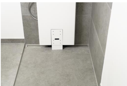
Picture 3: Suction inlet by floor (uni-drain)
