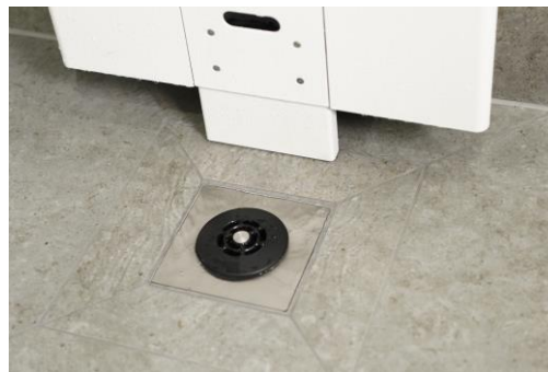
Picture 2: Suction inlet by floor (point drain)
